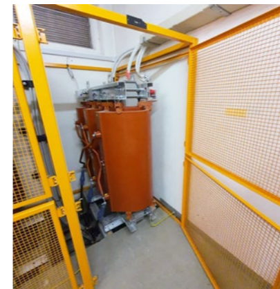
Trafostation Pumpstation: neuer Trockentransformator
